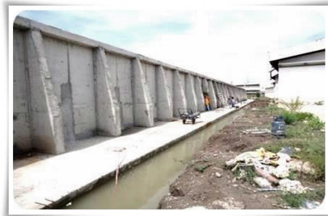
Fig. 2. Flood Protection (source: Industrial estate authority of Thailand, 2019)
